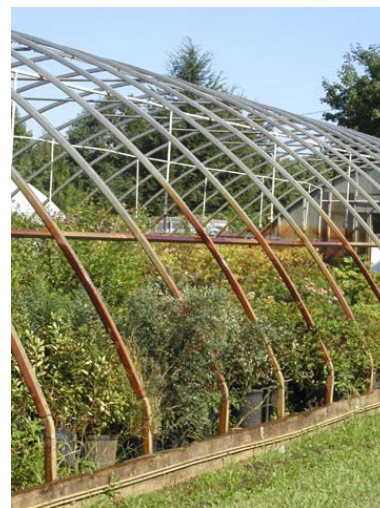
Fig. 2. Rusting of metal structures.
